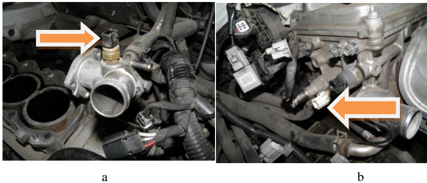
Fig.4.6. Features of the engine design (a, b – location of the temperature sensor on the outlet coolant pipe of the cylinder head), causing the temperature sensor to fail to respond to overheating in the event of an emergency loss of coolant [35]
